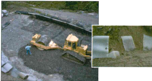
Fig. 5. Construction: first layers, fill compaction by heavy equipment, formwork, geogrids, drainage mats.
