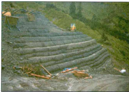
Fig. 6. Construction: partial view of the geogrid-reinforced slope. Note the "bellies" of the first layers.
