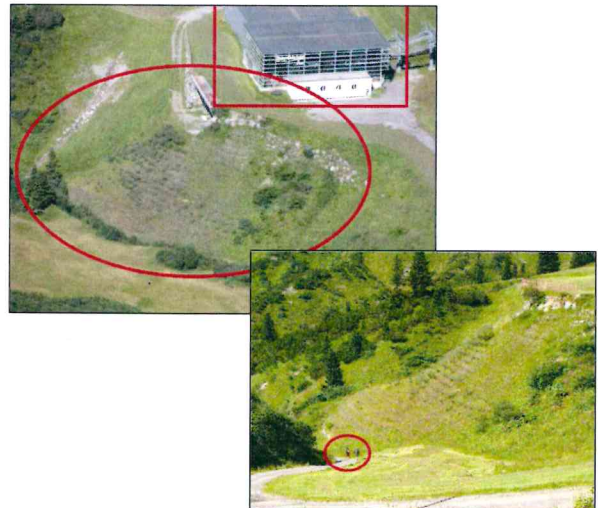
Fig. 9. August 2014: left up: overview, reinforced slope is marked; right down: persons as a scale for the structure.
