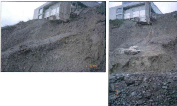
Fig. 3. Part of landslide with endangered lift station.
